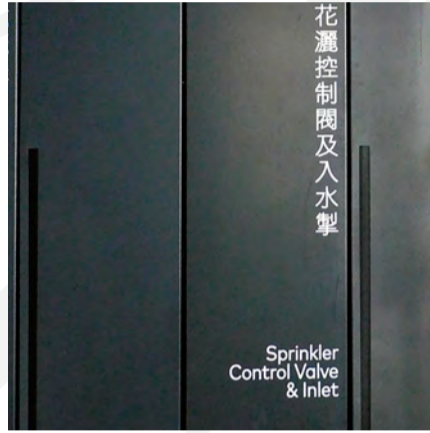
+ Fire control room
